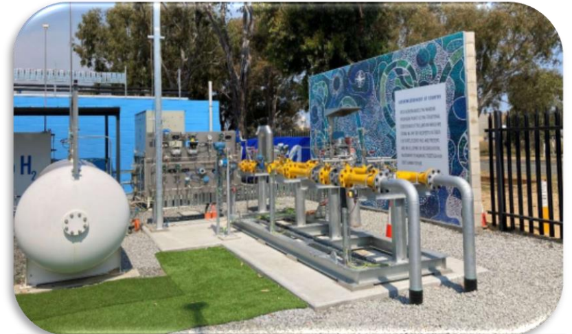
ATCO Gas Blending Project
